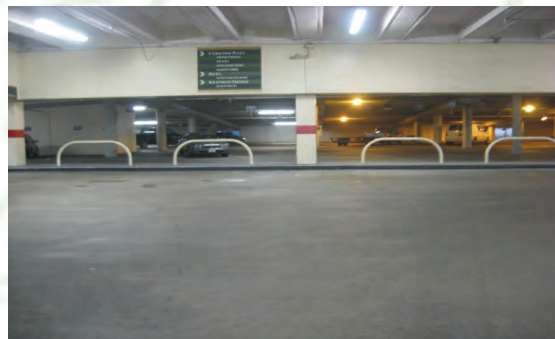
Garage lighting retrofit improved color rendering index scores & supports the LEED energy & atmosphere credit by improving the scoring potential for ENERGY STAR rating. (Left: new lighting, Right: old
